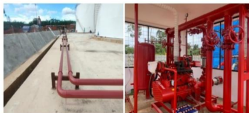
System Hydrant 6 x 1500 KL
